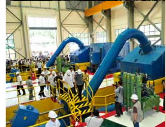
Sibulan Hydro Power Plant
