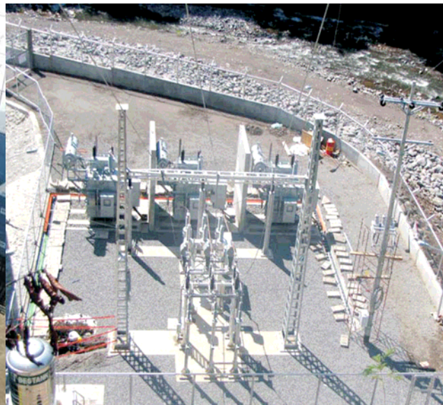
Powerhouse B Substation
